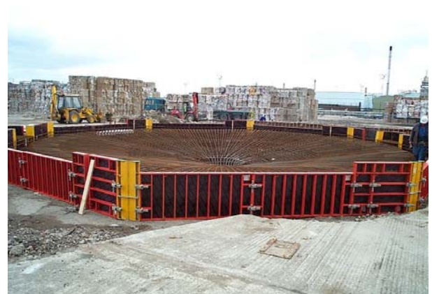
22 m diameter Clarifier
